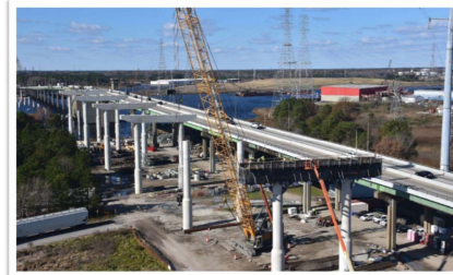
PICTURE 3 – Construction of the High-Rise Bridge for the HRBT Projects. (Source: VDOT)
